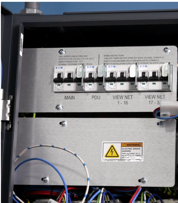
Breaker cover panel
