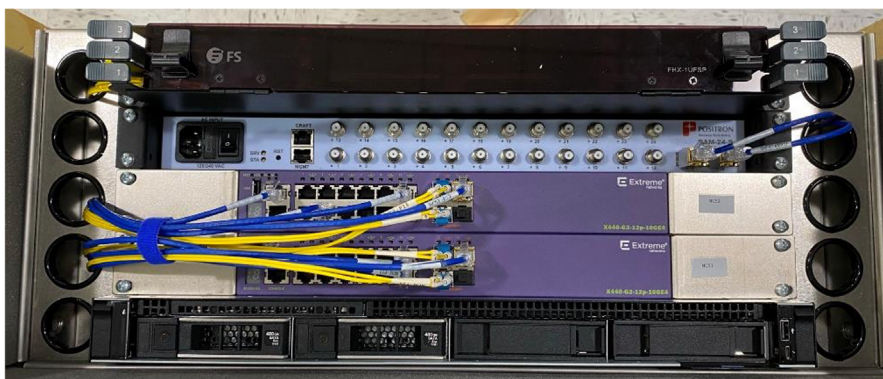
iNode Server mounted in Telco rack
