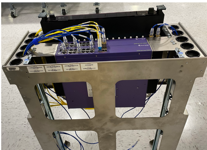
Telco Rack Ready for Install in Control Panel*
