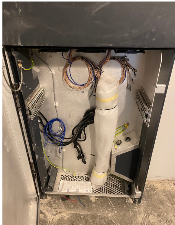
CP 5.0 Lower Section for TELCO Rack
